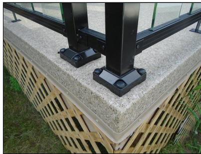
1.3 Item 2(Picture) Top mount railings are vulnerable to water penetration
