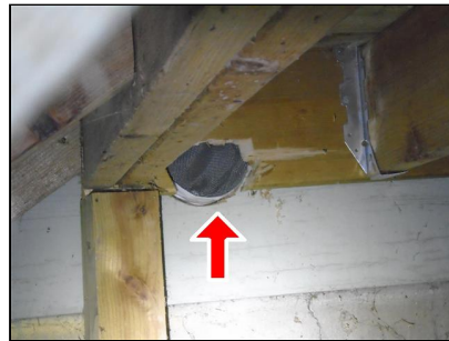
4.4 Item 4(Picture) Kitchen vent termination is under the deck
