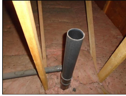
8.0 Item 1(Picture) Plumbing vent
