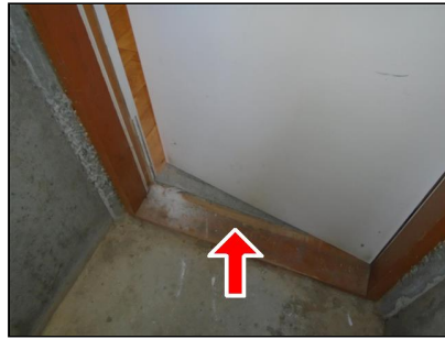
1.1 Item 1(Picture) Basement entrance (rubs at the bottom)
