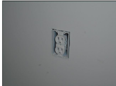
6.3 Item 7(Picture) Multiple boxes in basement
