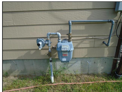
8.6 Item 1(Picture) Gas meter
