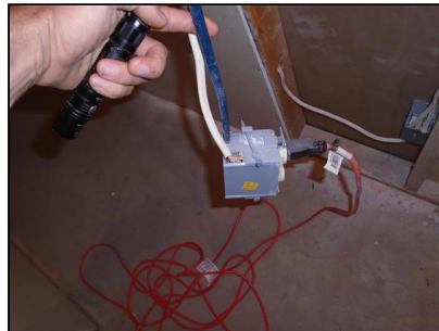
6.3 Item 4(Picture) Under stairs. This receptacle is also using an extension cord going to a freezer
