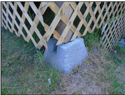
1.3 Item 1(Picture) Improper footing (not frost protected)
