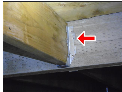
1.3 Item 3(Picture) Improper fasteners in joist hanger
