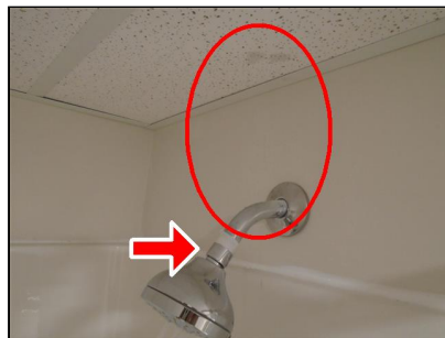
8.2 Item 2(Picture) Basement shower is spraying on the wall and ceiling behind.
