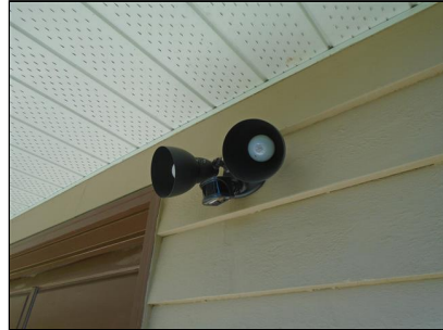
6.3 Item 3(Picture) Lights connected to garage cord (item 2)
