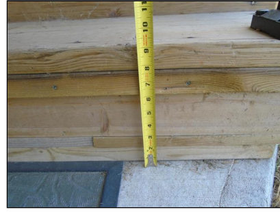
1.3 Item 6(Picture) Uneven step (refer to item 7)
