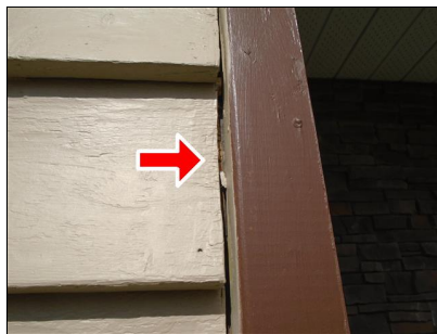
1.0 Item 2(Picture) All corners should be caulked
