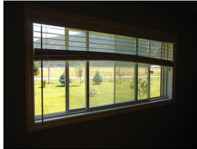
9.6 Item 1(Picture) Almost all windows
