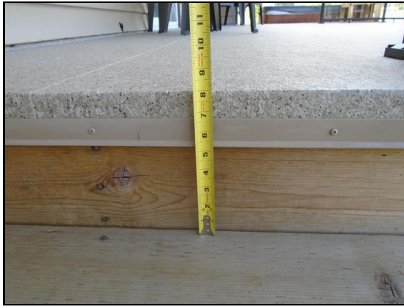
1.3 Item 7(Picture) Uneven steps are a trip hazard
