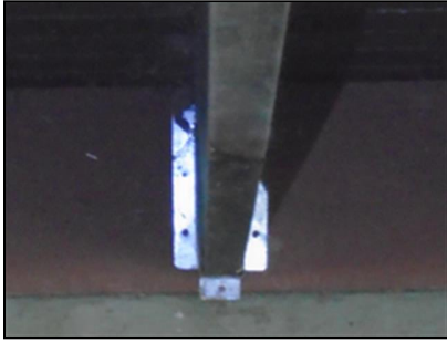
1.3 Item 4(Picture) Missing fasteners in joist hanger
