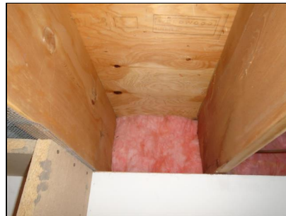
4.2 Item 1(Picture) Spaces between floor joists should be sealed
